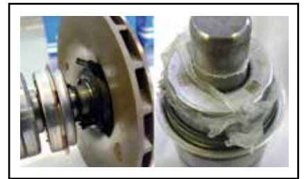
10.10 Improper use of sealing material
