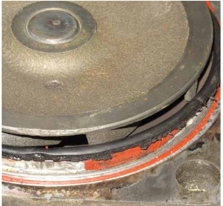
10.12 Sealant paste Sealant paste incorrectly applied on O-rings
