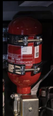
Fire extinguishing system
